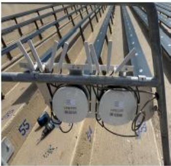
(b) APs mounted on a handrail.
